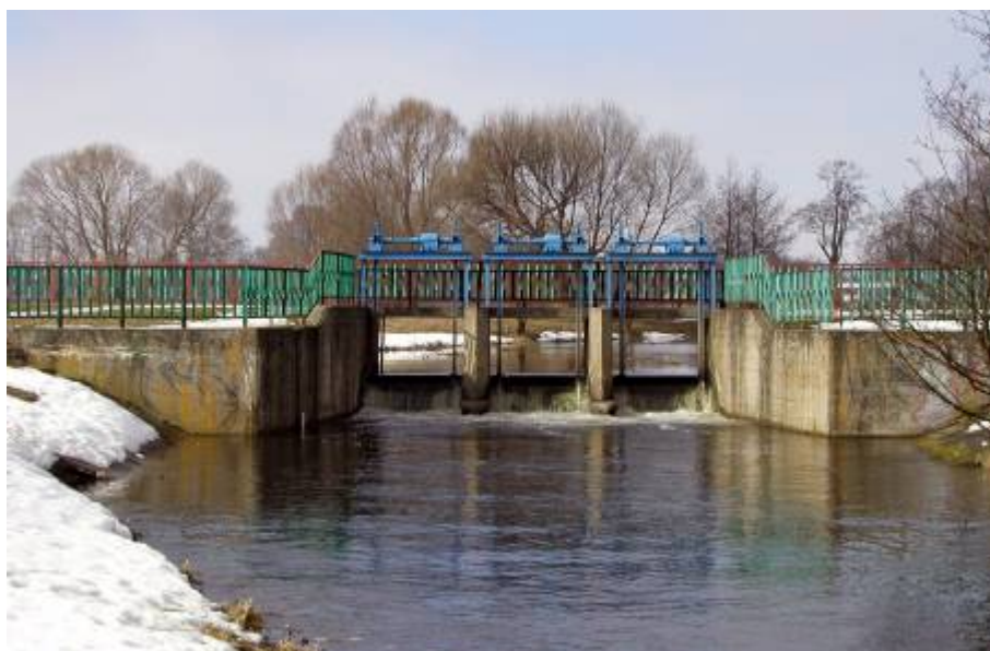
Phot. 4. Weir on the Black Hańcza ( photo by R. Kujawa )
