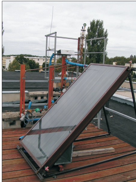
Fig. 1. Experimental solar installation on the roof of building
